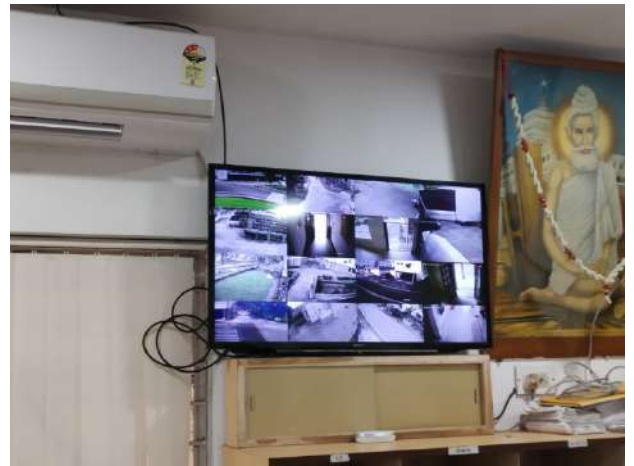
CCTV camera monitoring facility in the office.
