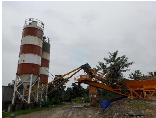
Fig. 7 Silos for Base-Subbase Material Storage
